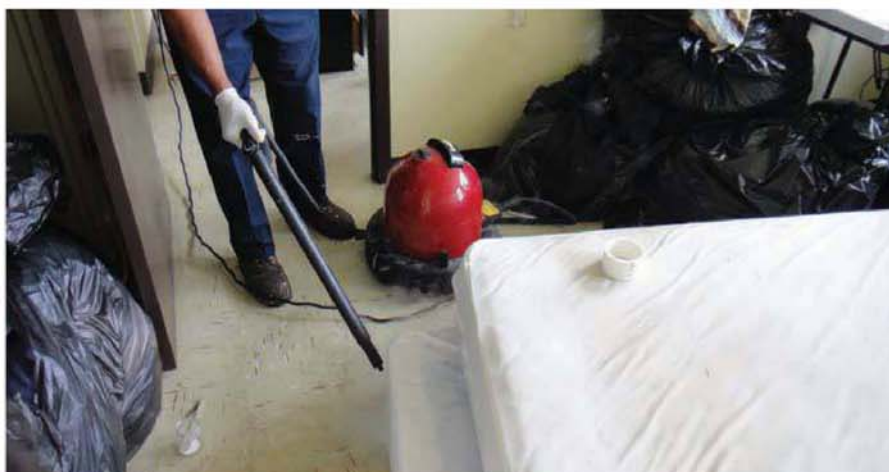
Applying steam to mattresses and box springs is an effective and safe control method.
